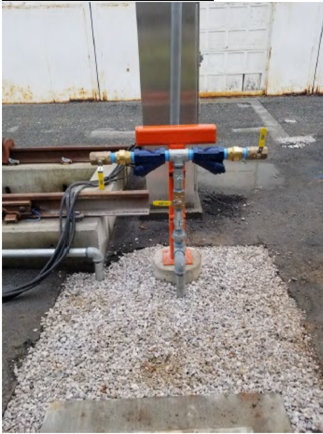
New Compressed Air Connection
