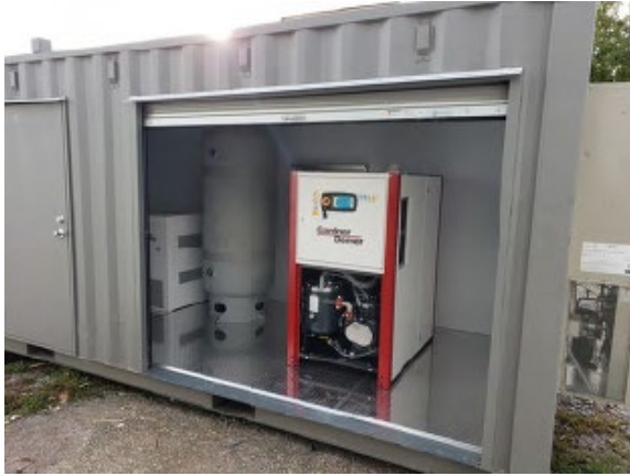
New Compressed Air Plant – Interior
